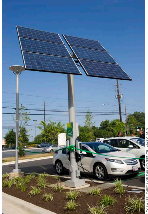
Tracking solar array to charge electric cars.
