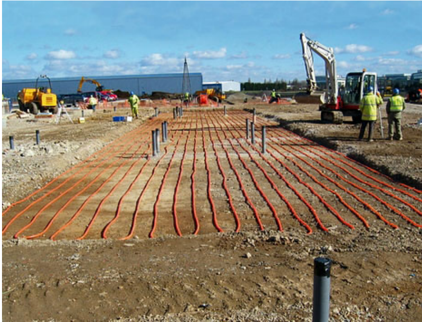
Figure VII-17: Thermal bank pipe being laid at Howe Dell School (Britain). Source: ICAX ThermalBanks 2016. Courtesy of ICAX. Copyright ICAX www.icax.co.uk
