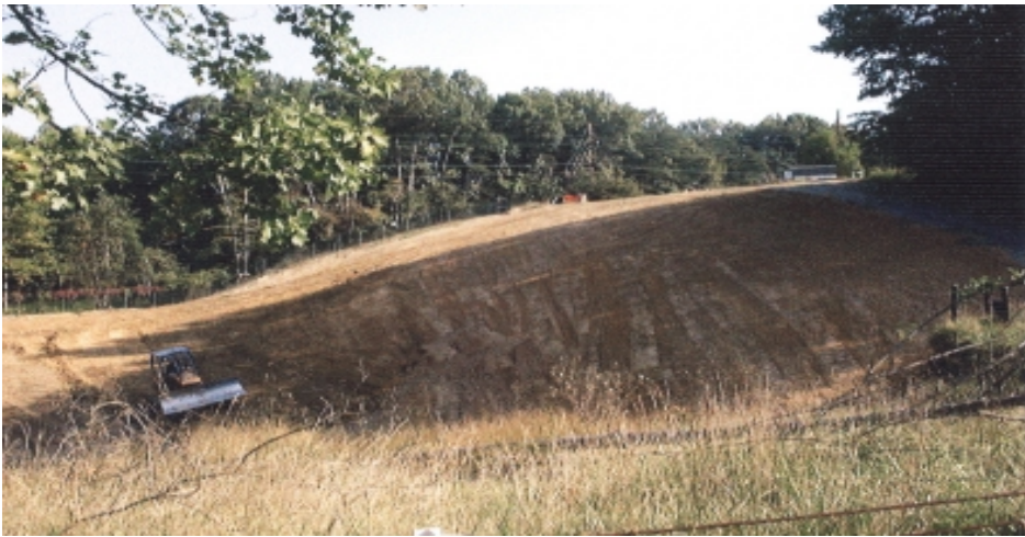
Above an earth mover grades the old Site 3 landfill after its cleanup at the former Naval Surface Warfare Center-White Oak near Silver Spring.
