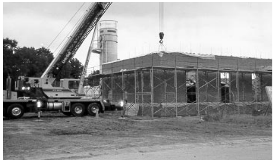
Town of Delmar's new water treatment plant. The entire community anticipates the project completion by the end of the year.
