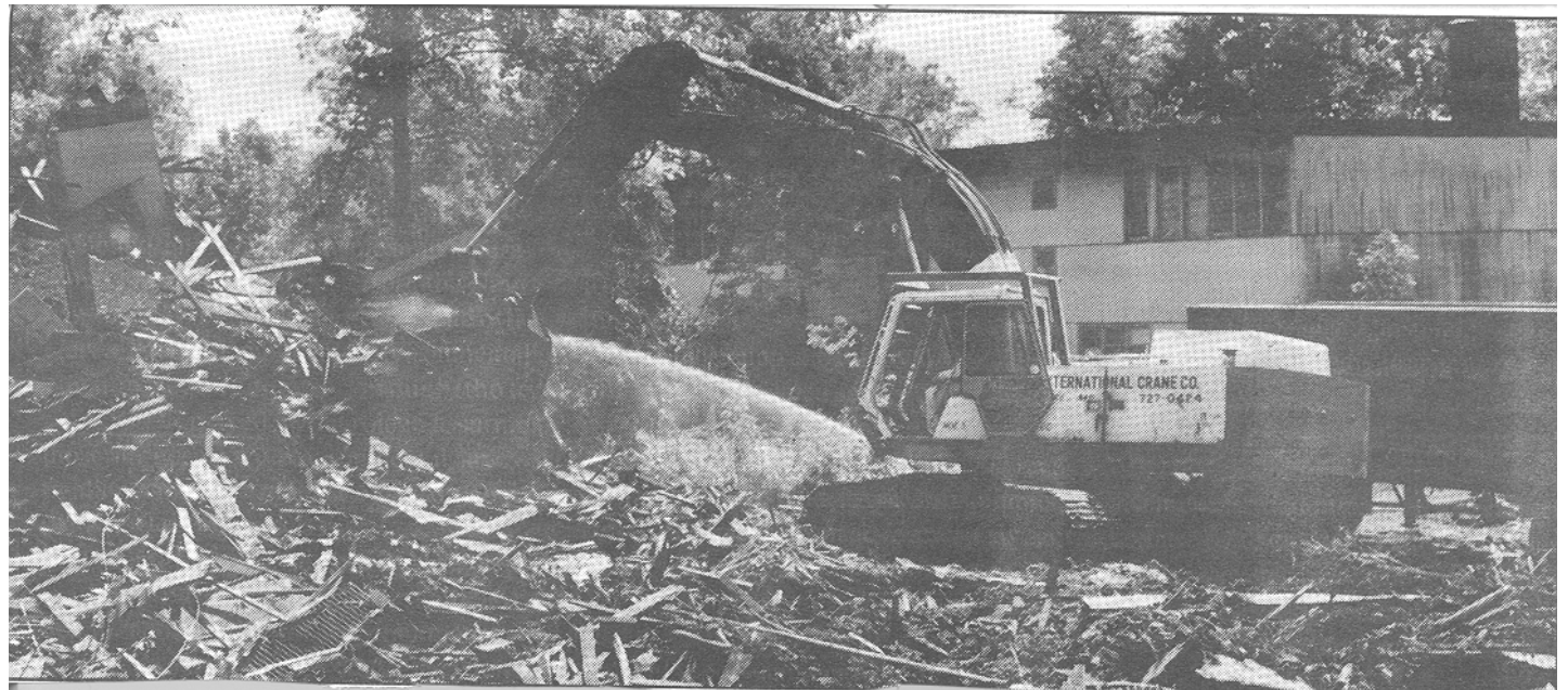
A crane clears debris from an area at the Naval Training Center-Bainbridge in Cecil County.
