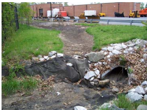
Figure 3-13 Failed Bioretention at SHA Glen Burnie Maintenance Shop
