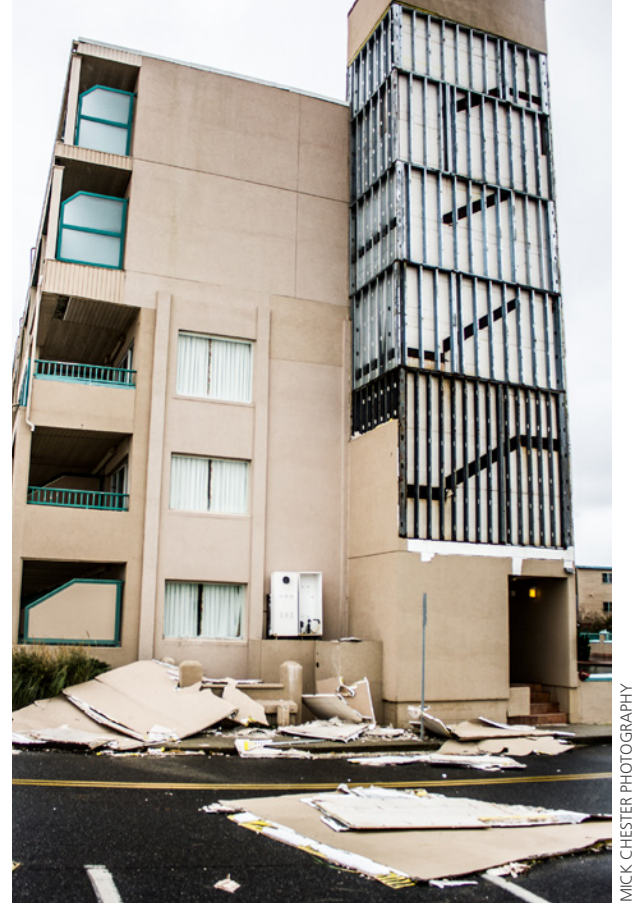
Building damage in Ocean City following Hurricane Sandy.
