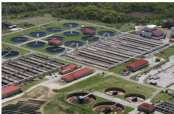
Black River wastewater treatment plant near Baltimore, Maryland (Jane Thomas, IAN, UMCES)
