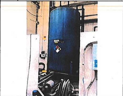
Photo #5: Tank #643 used for the storage of PCB wastes 0-49 ppm.
