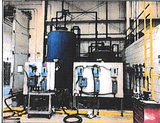
Photo #4: PCB waste storage tanks.
