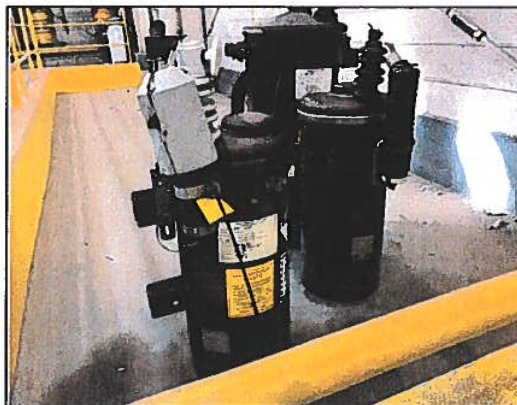
Photo #8: PCB waste storage area for drums and transformers.
