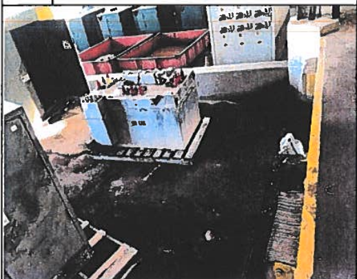
Photo #11: Transformer storage within the loading/unloading bays.
