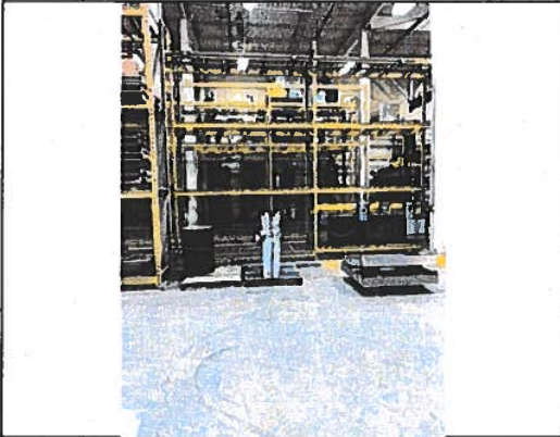
Photo #3: Storage area for PCB wastes (transformers).
