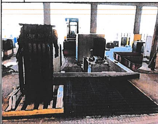
Photo #12: Transformer storage on the drainage grate to the vaulted AST.
