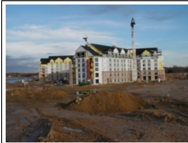
Work continues on the Hyatt Regency Chesapeake Bay Resort, Spa & Marina complex in Cambridge, a project of the state's Voluntary Cleanup Program.
