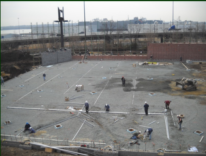
Example SSDS Installation
