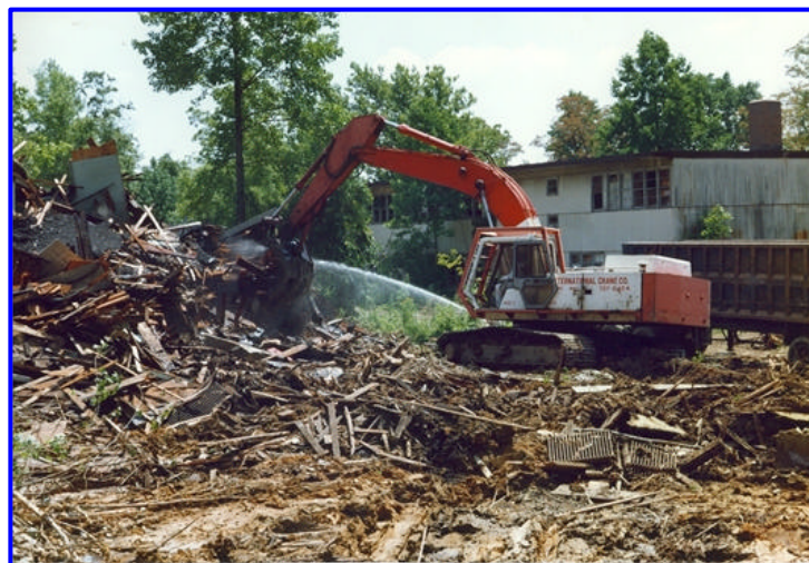
An excavator clears debris at the Naval Training Center at Bainbridge in Cecil County.
