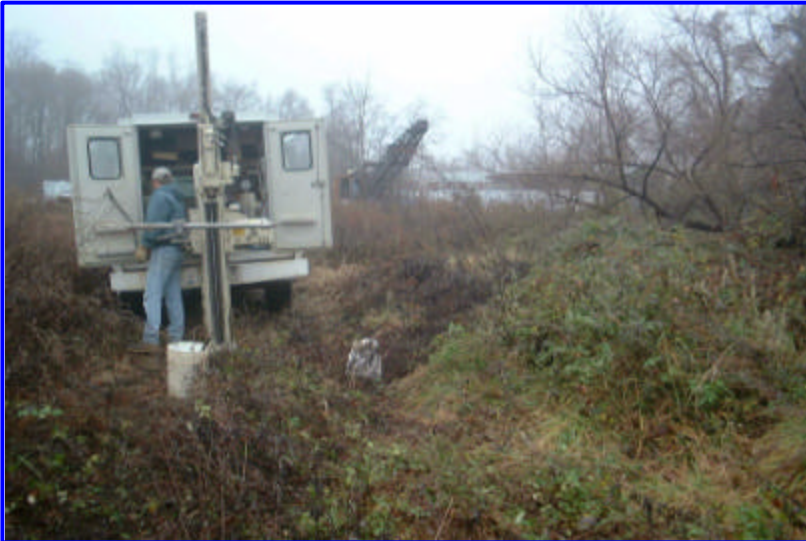
Direct push technology used to collect soil and groundwater samples at the Sauer Dump Site, Baltimore County, MD.
