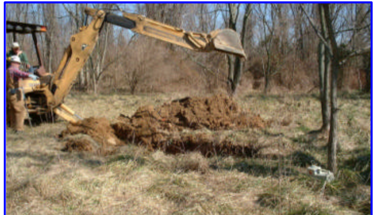
Test pit excavation at the Contee Sand and Gravel site in Prince George's County, MD to investigate the presence of hazardous waste in the landfill.
