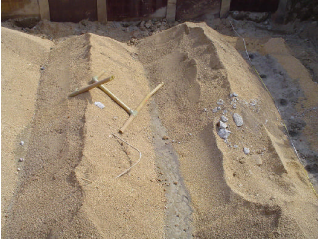
Photo 9 - View of tankfield following UST removal facing northeast. 10K UST centerline to right of photo, 8K UST centerline to left of photo.
