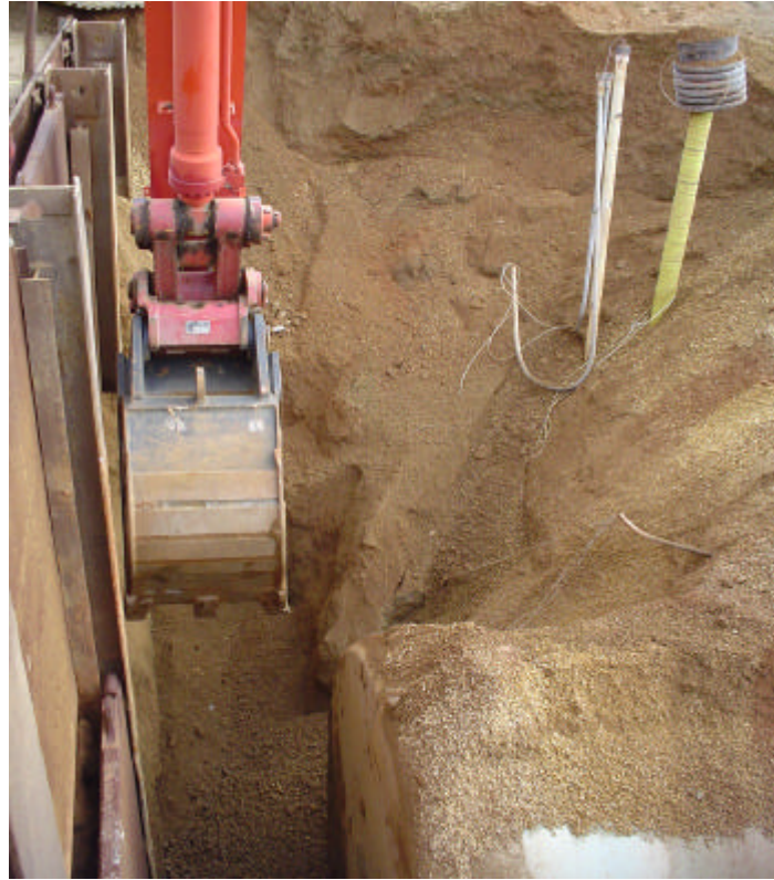
Photo 1 - View of excavation for shoring installation. North end of 12K UST in foreground.
