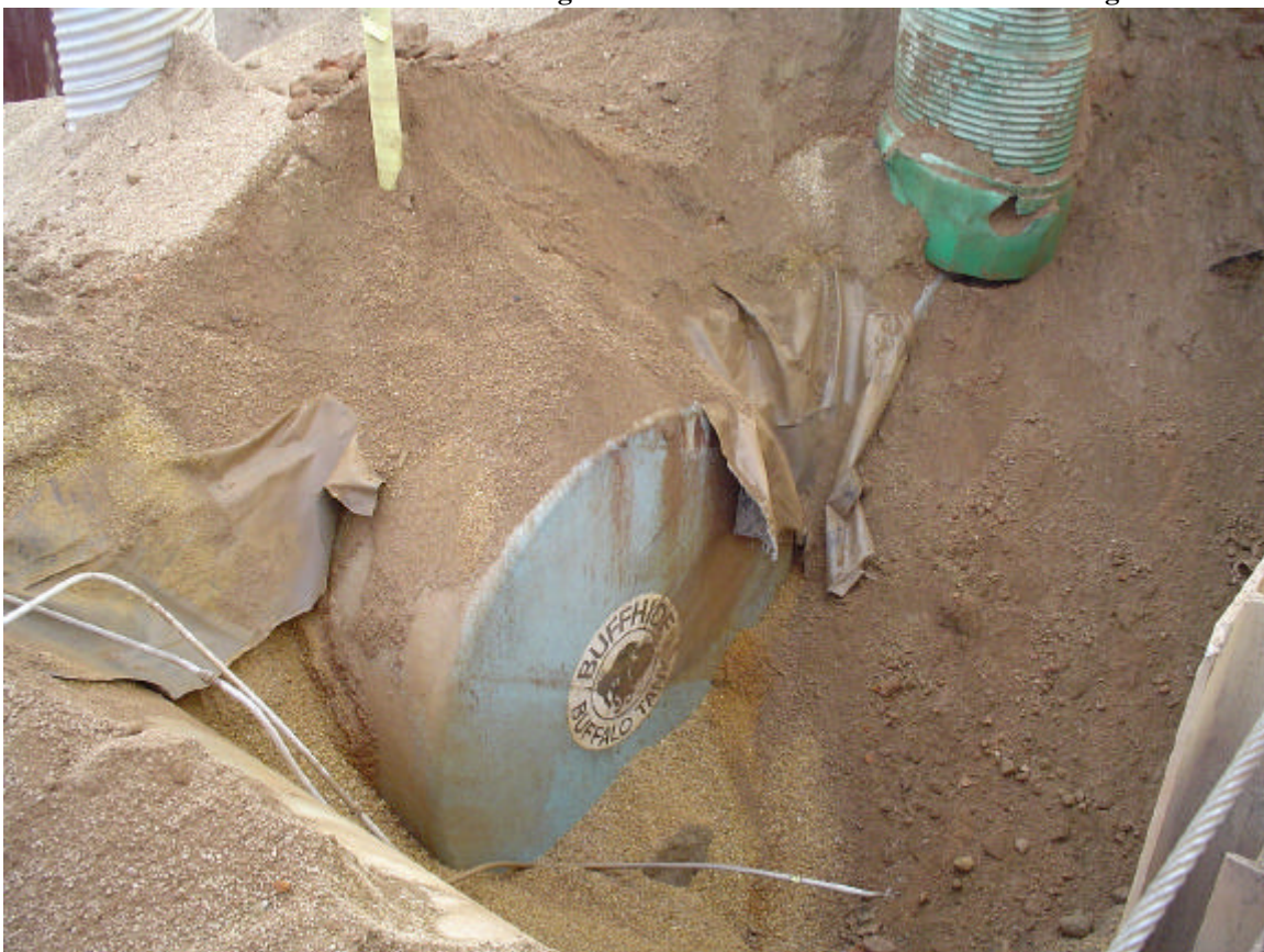
Photo 2 - View of excavation for shoring installation. South end of 8K UST in center of photo.
