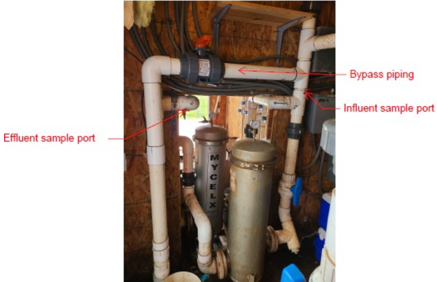
Photo 1: Influent and effluent sample ports as well as bypass piping.
