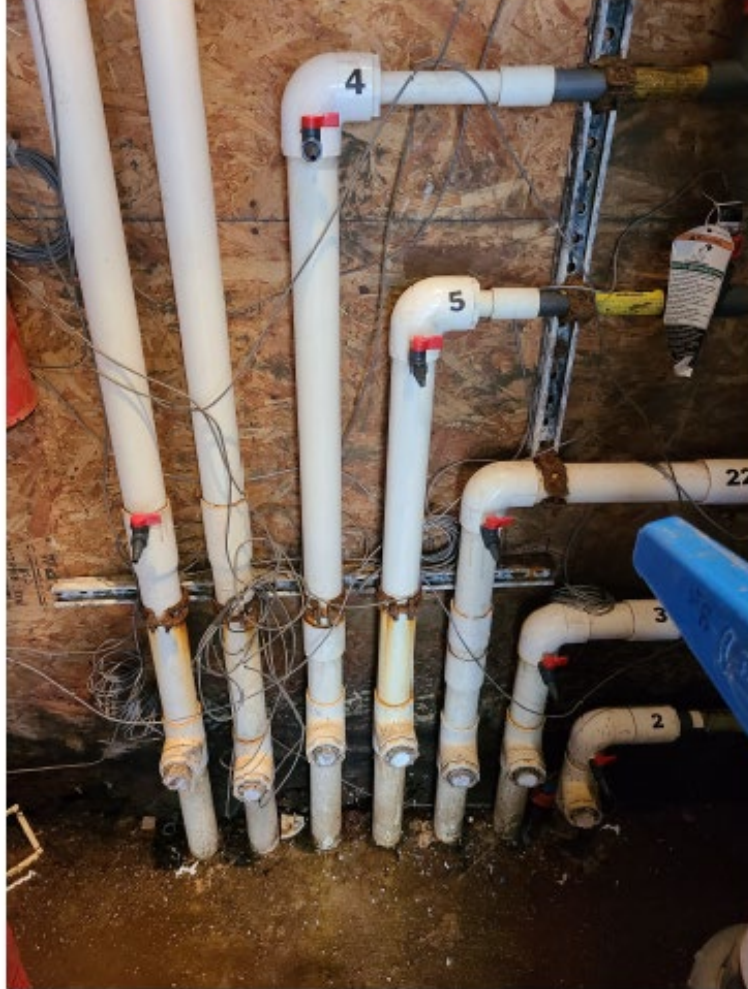
Photo 3: Sample ports installed on influent lines from each recovery well.
