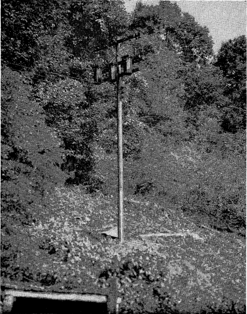
New transformer arrangement at Castle Mine, Big Vein Coal Company of Lonaconing, Inc.
