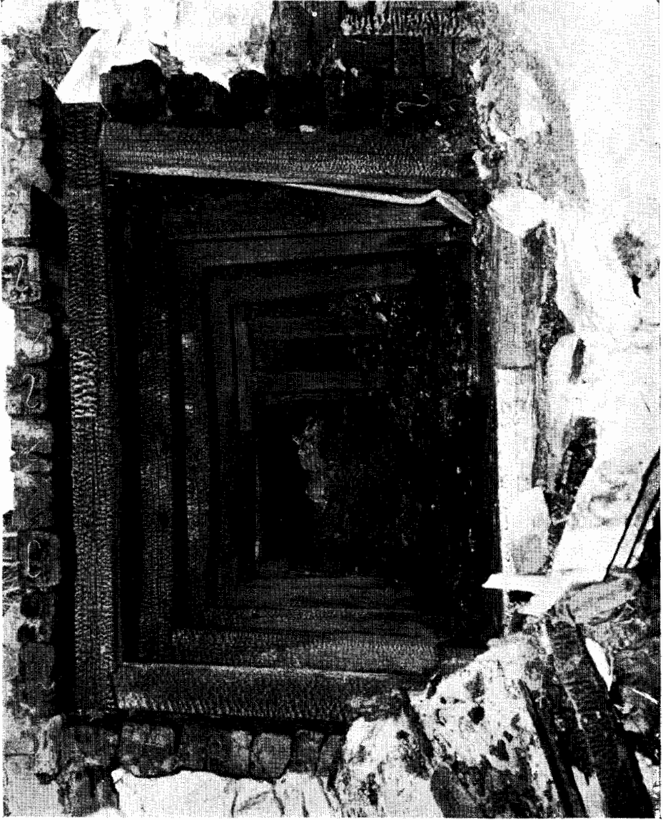
Mitt No. 1 Mine showing charred timber.
