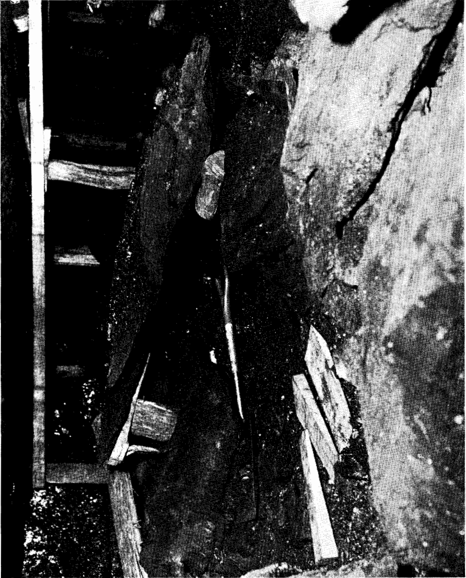
Scene at Hamill Mine, McNitt Coal Co., where Wolford Richard Prando was killed by a fall of rock.
