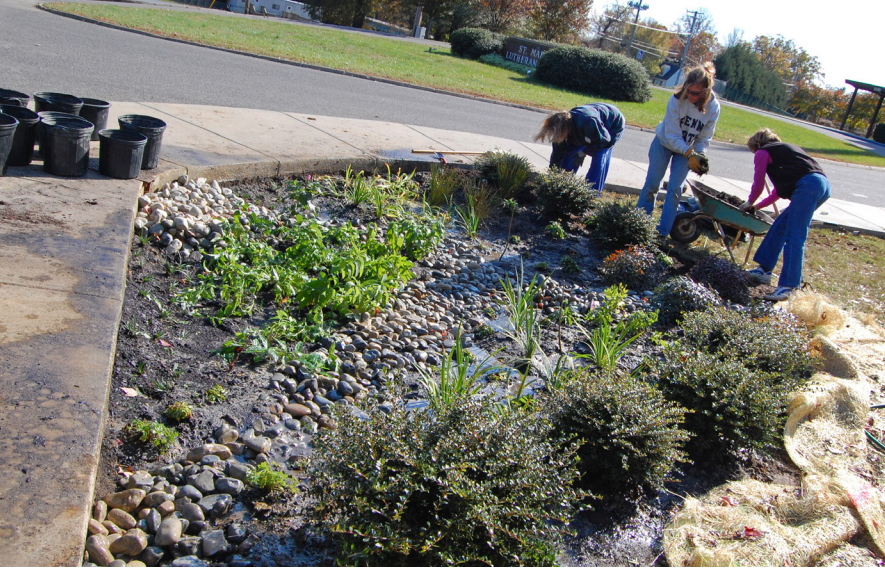
Many new developed rain gardens greatly aid stormwater in soaking into the ground.
