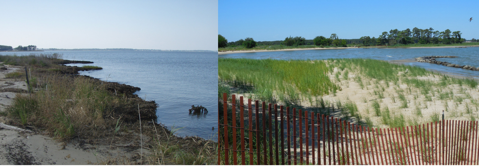
The rehabilitation of the coast line at Ferry Point Park in Kent Narrows over a five-year period is a great example of planning and construction techniques that adapt to climate change.
