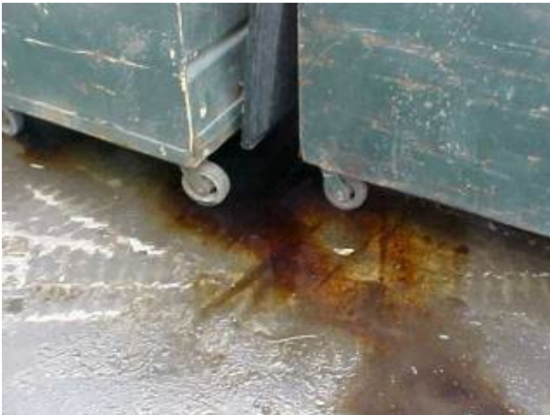
Figure 18. Example of visual observation indicating stormwater discharge exposed to pollutants.
