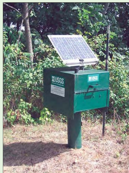
Observation well WA Ci 82 in Washington County, Maryland, with near-real-time transmission equipment. (Photograph by Charles J. Strain, USGS)
