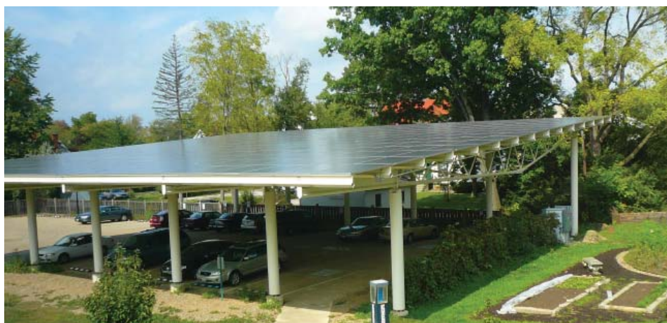
Figure 5-2. This parking lot at Oberlin College in Ohio is shaded by solar panels which generate power for the adjacent building, Credit: Nicole Stern
