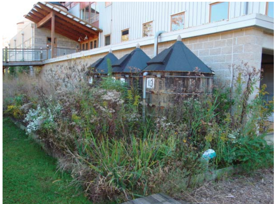
Figure 2-1. Rainwater Harvesting Cisterns at the Chesapeake Bay Foundation Building, Credit: Jennifer Dowdell
