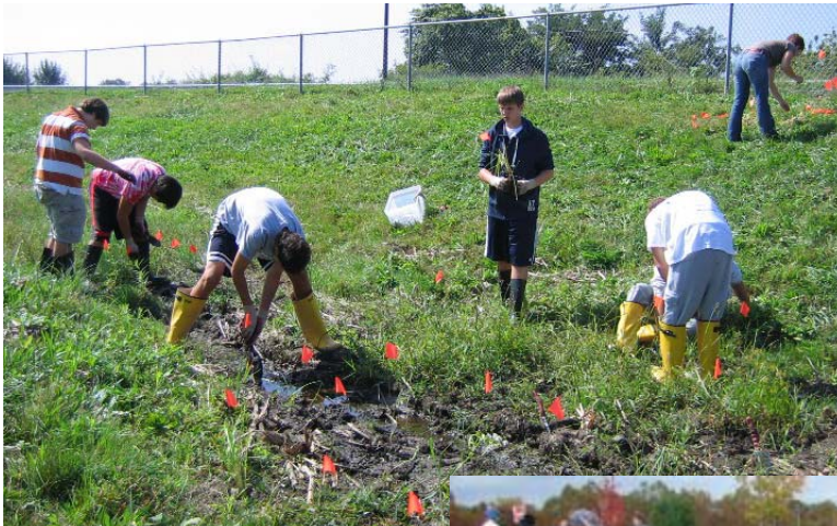
Left. Students at Urbana High School volunteer to place wetland plants in another 319(h) Grant-funded wetland creation demonstration project September 2010. In this project, 95 students from four classes learned about the value of stormwater management and wetlands. The hands-on experience reinforced their new understanding.
