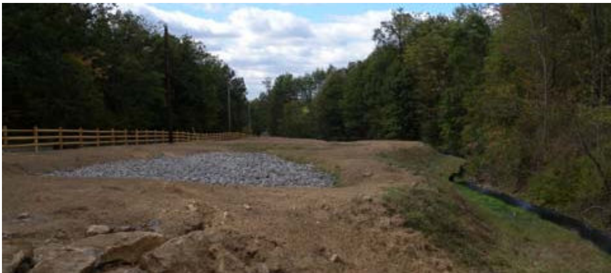
Figure 3. In 2010, construction was well underway on limestone leach bed and wetland mitigation portions of the Aaron Run acid mine drainage remediation project. (source: MDE Abandoned Mine Lands Division).
