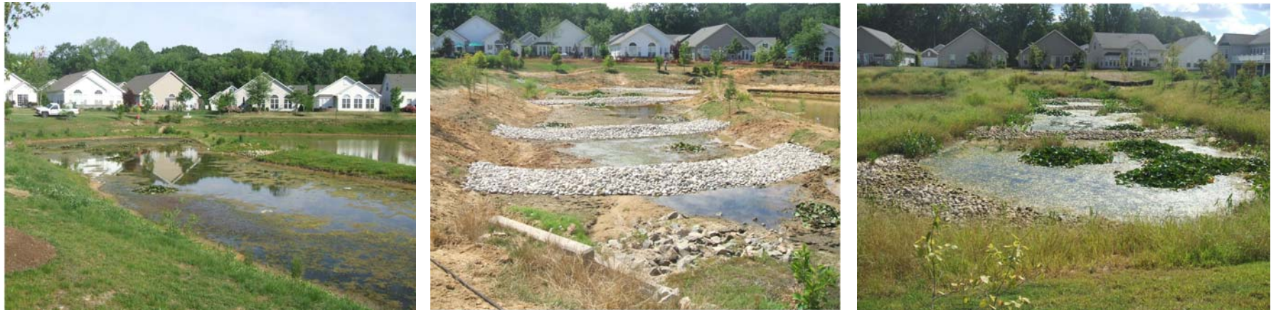
Figure 10. Corsica River Stormwater Management Retrofit at Symphony Village. The photographs above show before construction / during construction / after construction in a project by the Town of Centreville and the Maryland Department of Natural Resources that successfully converted a two-cell conventional stormwater retention pond into a multi-cell pond/wetland complex that improves water quality and habit diversity in the planned community of Symphony Village. (photos by Eva Kerchner, Corsica River Watershed Manager, Town of Centreville)
