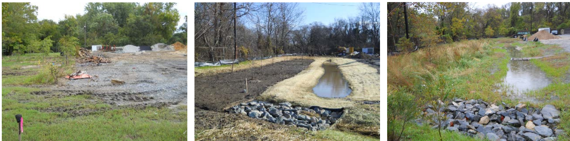
Figure 13. In the Town of Centreville, stormwater runoff from the Department of Public Works facility previously flowed overland across a materials staging area directly to the Corsica River (flowing right to left in the photos). To help protect the River, the edge of the materials staging area in the riparian zone (left) was converted in late 2011 to intercept runoff from the majority of the facility in a bioretention site (center). Project design and construction was supported in part by FFY2009 319(h) Grant funds. During Super Storm Sandy in late 2012, the bioretention site functioned as designed and maintained stability of the riparian zone (right).
