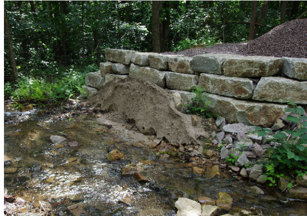
Figure 9. The AMD mitigation projects in the Casselman River watershed are demonstrating the application of limestone “sand” as an effective technique that offers low operation and maintenance cost compared to other approaches. The project constructed access sites at the stream bank where a truck deposits crushed limestone (left). Then, over time, the limestone particles roughly the size of sand washes into the stream and distributes downstream where it buffers in-stream acidity (right).
