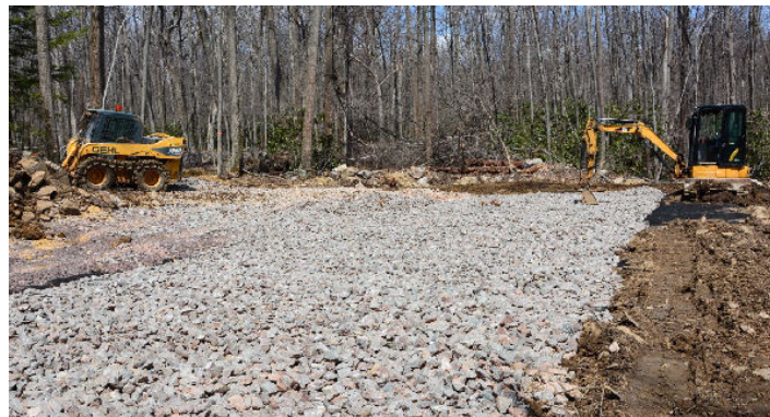
Figure 10. Some Casselman River watershed AMD mitigation Phase 1 sites employed excavation & construction of limestone leach beds (left). Upon completion of the leach bed (far left), acidic waters are directed thru the limestone to raise the pH level before the it reaches the stream. (Casselman photos by MDE Abandoned Mine Land Division.)
