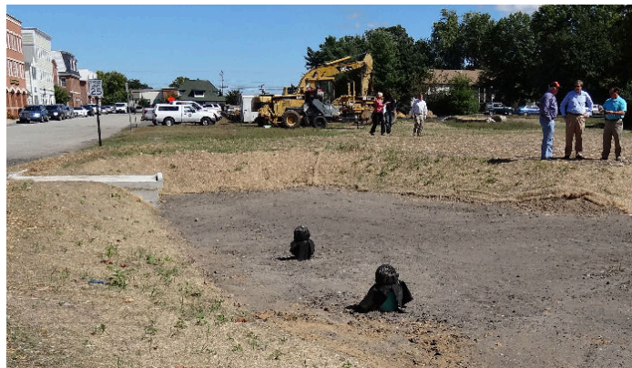
Figure 14. In Sept 2013 near Centreville's historic rail road terminal, the Town Watershed Manager shows construction of a bioretention area to MDE and EPA staff (near left, photo by MDE). About a month later, the project is complete and functional with newly planted colorful vegetation. (far left, photo courtesy of Centreville)
