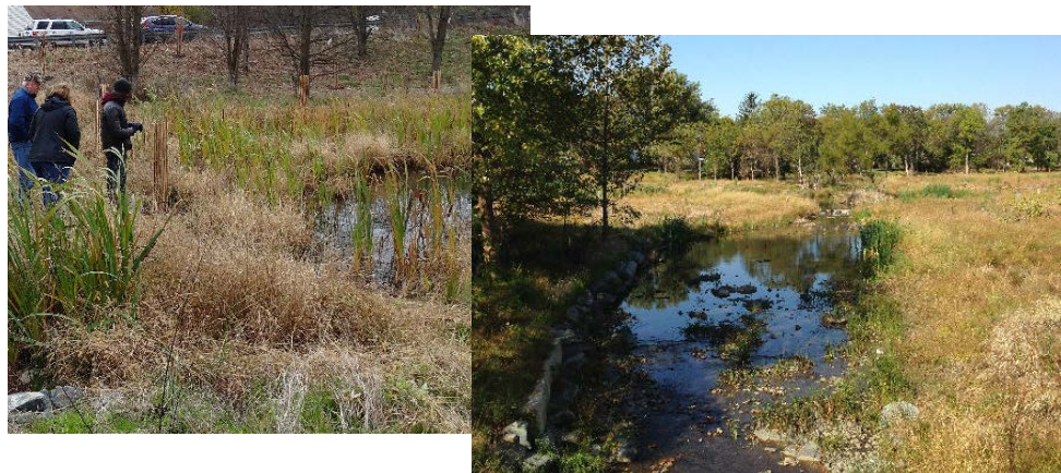
Figure 17. The completed Scotts Level stream restoration project eliminated the eroding stream banks, reconnected the stream to its floodplain and created wetlands. (far right). In November 2014, Baltimore County hosted EPA and MDE representatives at the project site. In the center-right picture, they are inspecting one of the created wetlands. (MDE photos)
