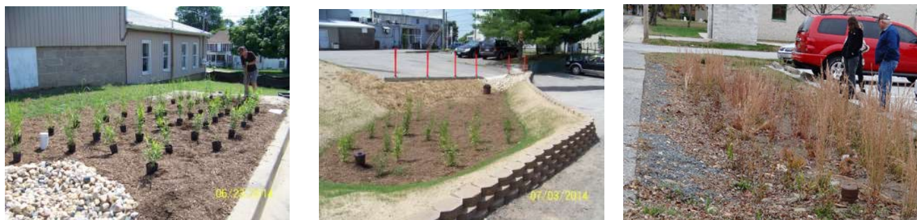
Figure 22. Caroline County used 319 Grant funds (FFY12 #6) to help complete construction of several projects to manage stormwater runoff in the Town of Greensboro during 2014. In June, plantings were being installed in a new stormwater infiltration area serving the Town Hall parking lot (left). In July, installation of a similar area was completed next to the Town’s Public Works Dept. garage (center). On November 13, 2014, Caroline County hosted EPA and MDE representatives who conducted on-site reviews of all the 319 grant-funds projects in Greenboro including the recently completed stormwater infiltration area serving the public library (right). (photos courtesy of Caroline County and MDE).
