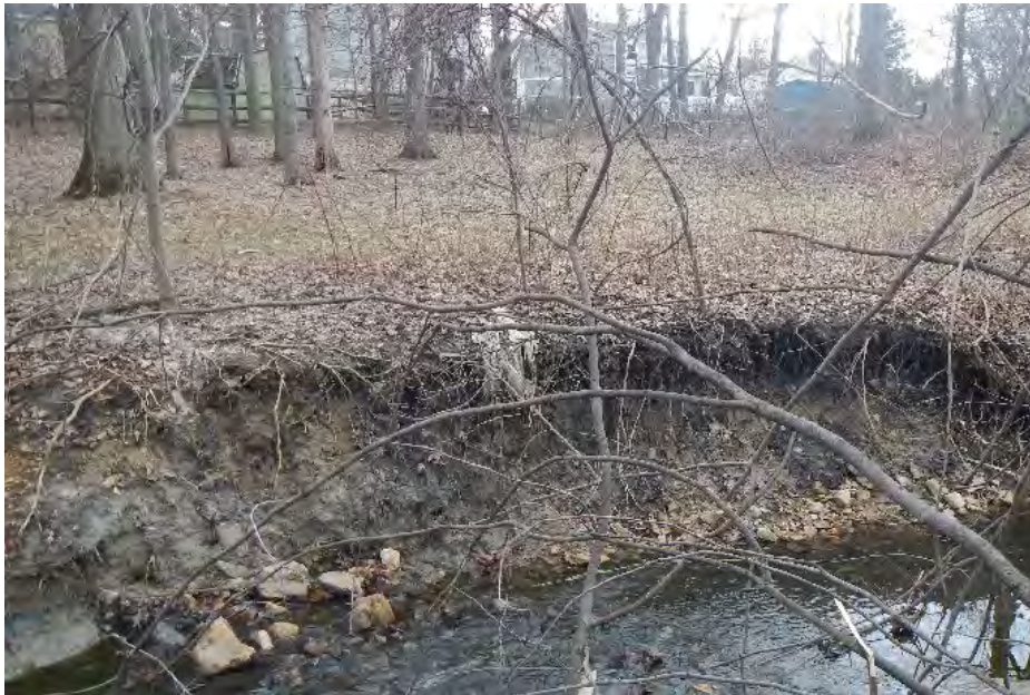
Figure 14. The two photos show existing conditions in the Scotts Level Branch drainage area in the vicinity of Marriottsville Road within the Middle Gwynns Falls watershed. A FFY2016 319(h) Grant for over $0.6M is scheduled to begin construction sometime next year to eliminate the eroding vertical stream banks and to restore the stream area. Total project cost is projected to be well over $1.0M. Project completion is projected before June 2019. (photo by Baltimore County Dept. of Environmental Protection and Sustainability, Capital Program and Operations Section).
