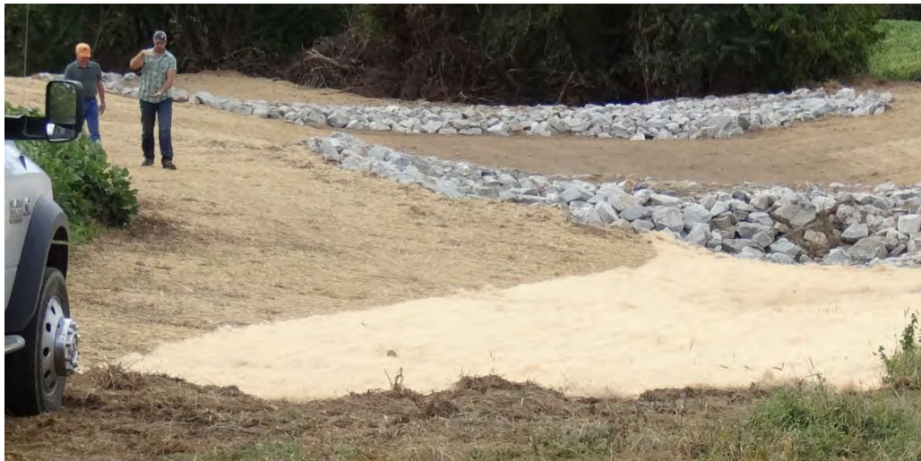
Figure 16. The photo above shows a newly constructed BMP on a Kent County farm as seen 9/26/17 when EPA and MDE representatives visited. The farm's steep slope and large drainage area required that grade stabilization be provided by rock. In between the rock, several bioretention/treatment wetland areas are ready for planting. Representatives in photo: Kent Soil Conservation District Board member, Sassafra River Association agricultural project leader. (photo by MDE, Integrated Water Planning Program)
