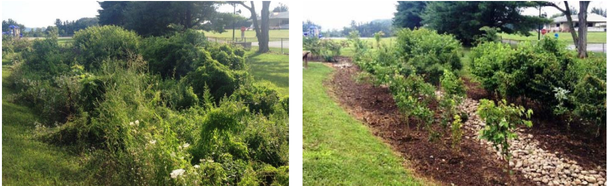
Figure 14. This summer at Frederick County's Urbana Elementary School, the bioswale presented maintenance issues common for some designs for this BMP. Invasive plant seeds are frequently entering the BMP and have the capability to overwhelm the native plantings in this type of design (left). After weeding (right) the extent of area needing intensive management is readily visible. This example helps illustrate how design selection determines long term maintenance needs and operational costs. (Map and photos are courtesy of Frederick County. Capital funding included 319 FFY08 project 4 completed 2012)
