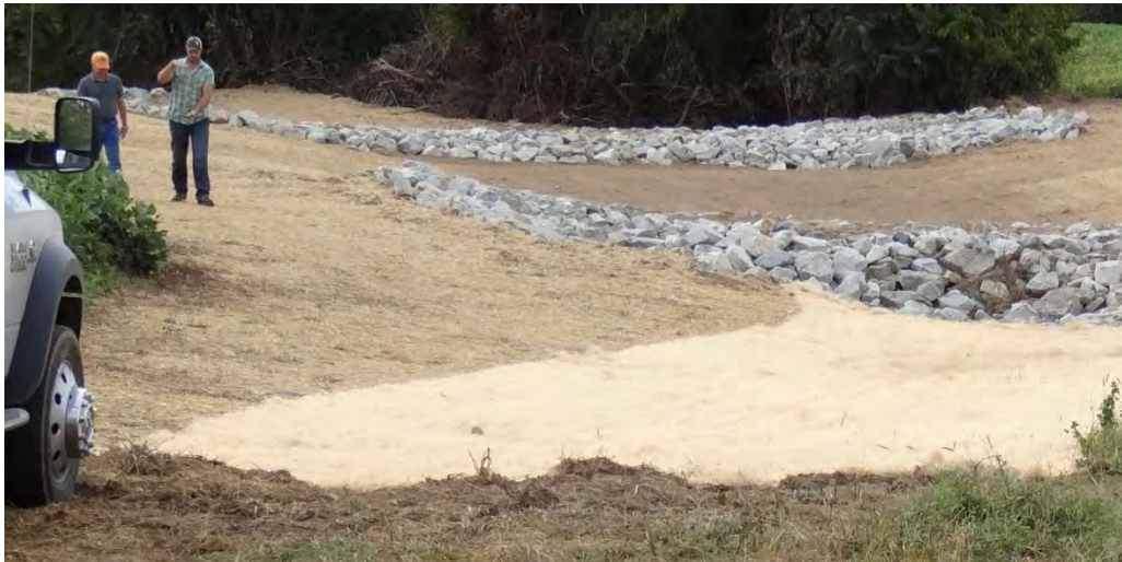
Figure 16. The photo above shows a newly constructed BMP on a Kent County farm as seen 9/26/17 when EPA and MDE representatives visited. The farm's steep slope and large drainage area required that grade stabilization be provided by rock. In between the rock, several bioretention/treatment wetland areas are ready for planting. Representatives in photo: Kent Soil Conservation District Board member, Sassafras River Association agricultural project leader (photo by MDE, Integrated Water Planning Program).
