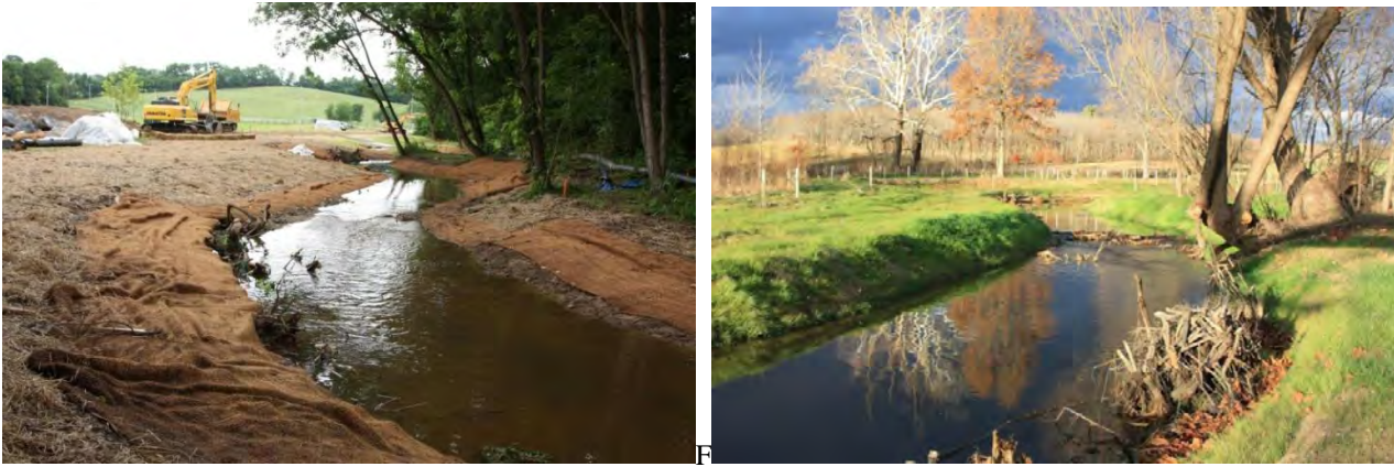
Figure 6. Stream restoration construction along Little Antietam Creek took place in 2016 (above left). Construction was completed late in 2016 (above right). The restoration was funded in part by two the 319(h) Grant in FFY2015 project #7) (photos by Washington County SCD).
