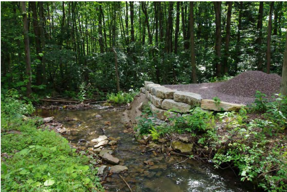
Figure 2. MDE’s Abandoned Mines Division hosted staff from EPA Region 3 at various acid mine remediation projects in the Casselman River watershed October 2018. The photo shows one of the sand-dumps funded in part by 319(h) Grant funds (photo by MDE).
