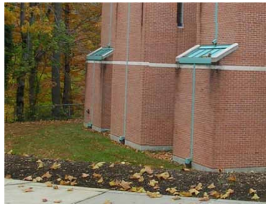
Direct connected downspouts suitable for disconnection at ISI site H-216
