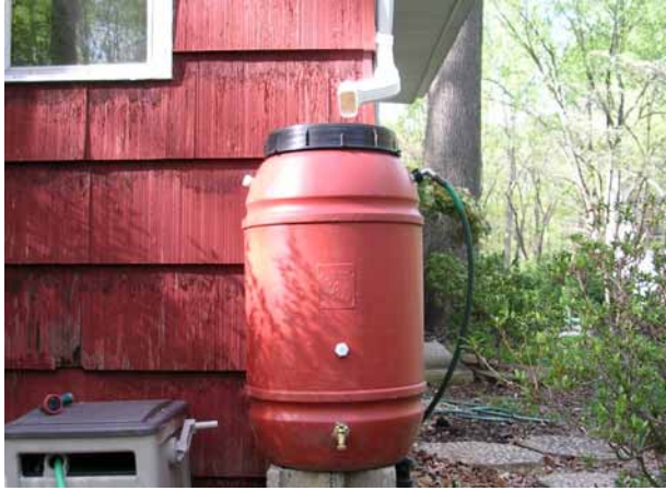
Typical rain barrel installation with overflow hose
