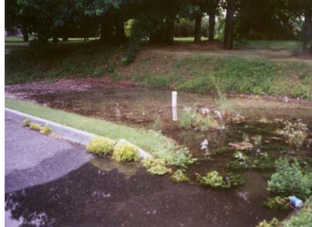
Figure 1: Failed Infiltration Trench
