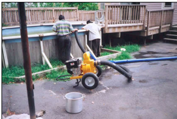
Figure 1: Swimming Pool Discharging to Street and into Storm Drain
