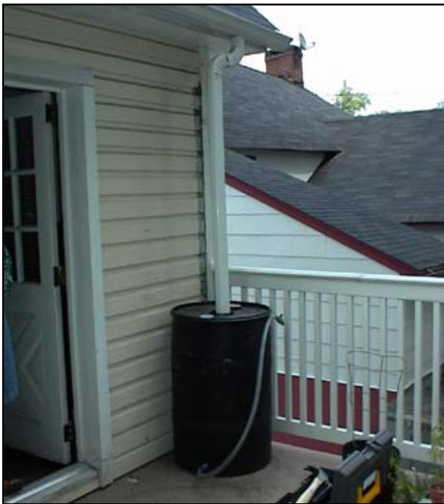
Figure 2: Rain barrel installed on a balcony due to space constraints on a small lot.
