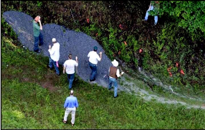
In an effort to prevent more flood damage to the Washington area, workers put gravel on a leak where water is sweeping through the dam.
