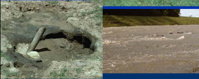
Hansen, 2007, Erosion of Earthen Spillways and Embankments
