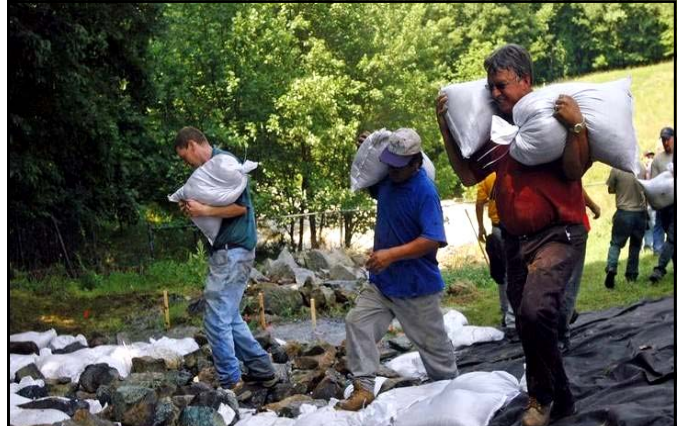
Area workers use sandbags as a temporary fix to stop the over flooding of the dam. Engineers and workers repair the damaged dam at Lake Needwood in Rock Creek Regional Park. The lake is 25 feet above normal and over 2,300 local residents were forced to evacuate.
