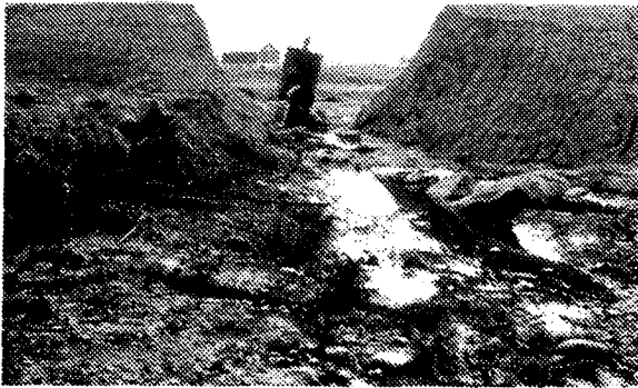
Earth Dam Failure
