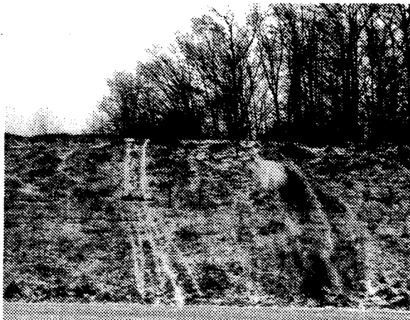
Damage to Slope
