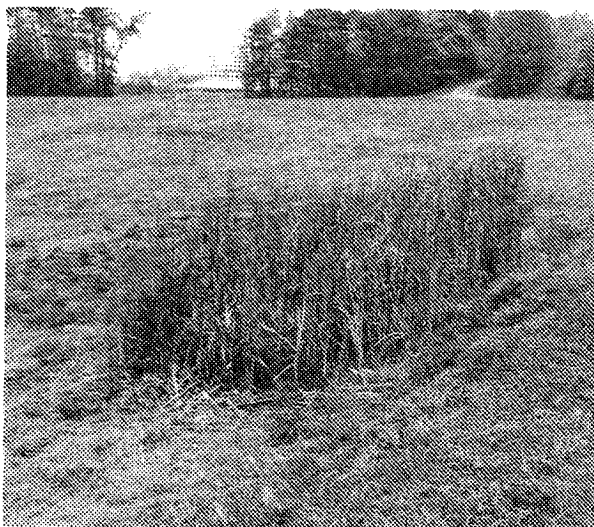
Evidence of Seepage
