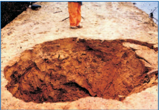
Sinkhole which developed over a spillway conduit.
