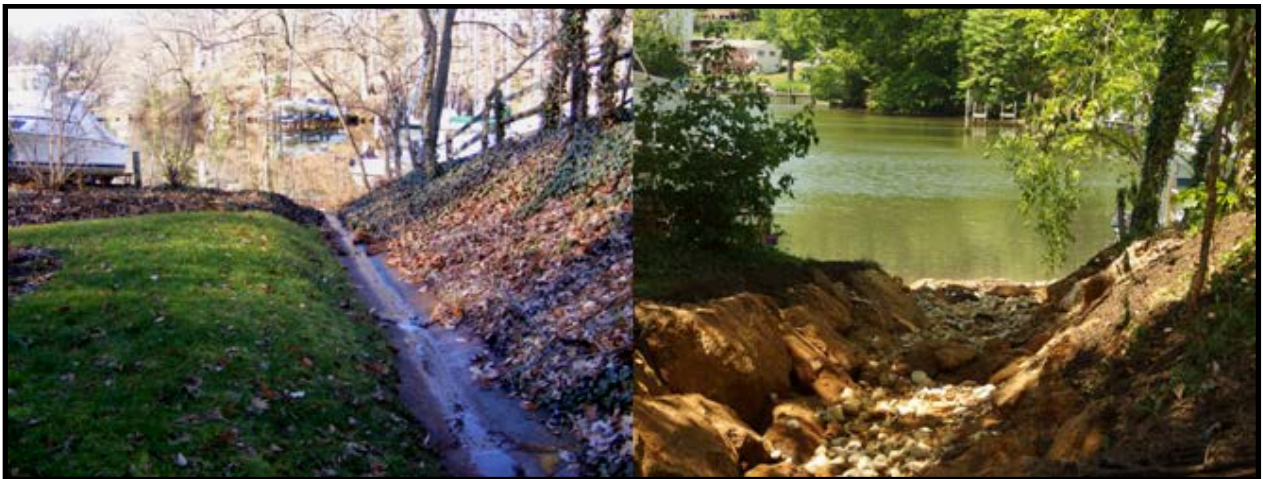
Figure 5: Outfall Stabilization - Anne Arundel County (Anne Arundel County WPRP)
