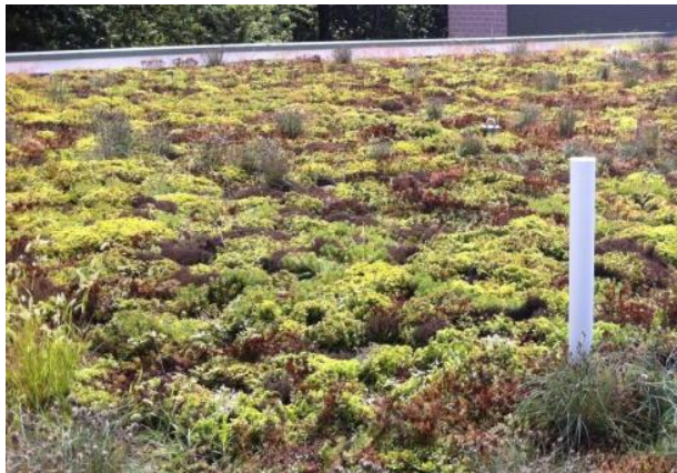
Green roof plants
