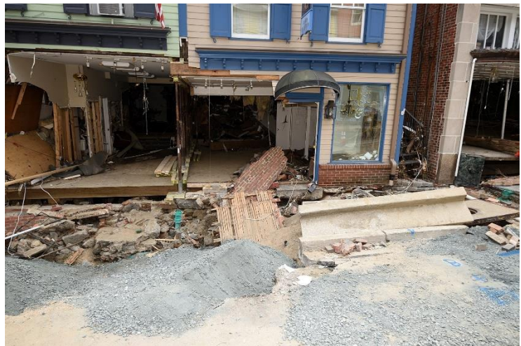
Flood damage along Main Street in Ellicott City on August 10, 2016. The suburban developments that have sprung up all around the town over the last 50 years have heightened flood risk during storm events by preventing natural drainage.
