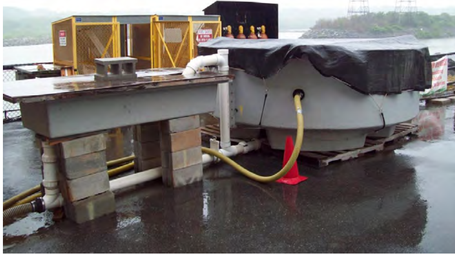
Photo 7. West Lift spawning tanks and related equipment.
