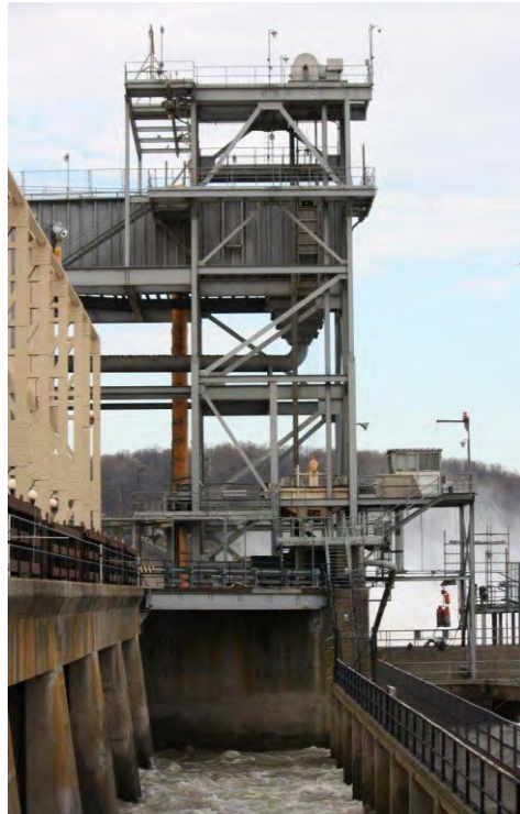
Photo 14. East Lift fish trough, attraction flow pipe, and hopper.
