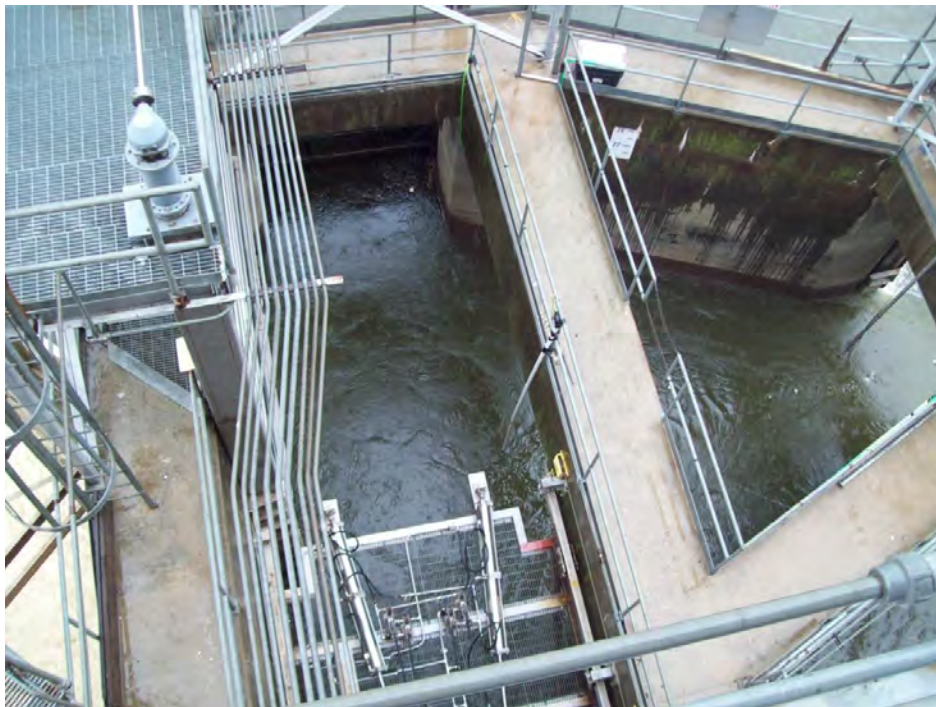
Photo 10. East Lift, plan view of Weir Gate "A" (right) and Weir Gate "B" (top).
