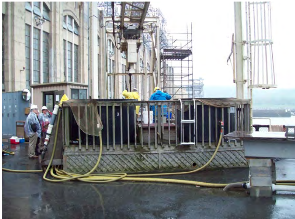
Photo 6. West Lift collection and sorting tanks.
