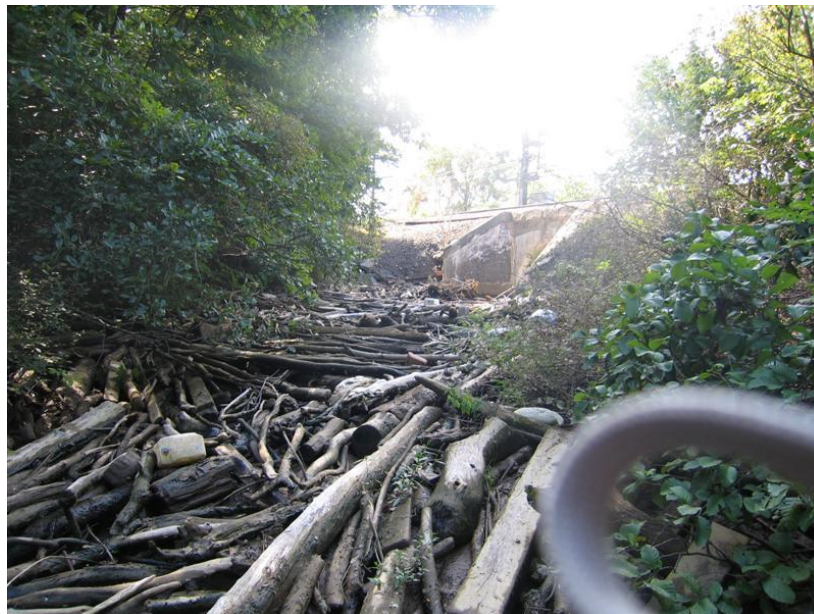
FIGURE 4.3-2: DEBRIS WITHIN TRIBUTARY. RAILROAD CULVERT IN BACKGROUND (SEPT 2007)
