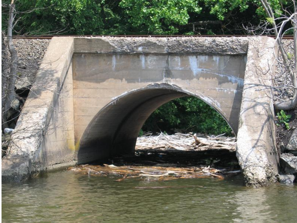
FIGURE 4.1.1-5: DEBRIS COLLECTING AT A RAILROAD CULVERT OUTLET (JUNE 2008)
