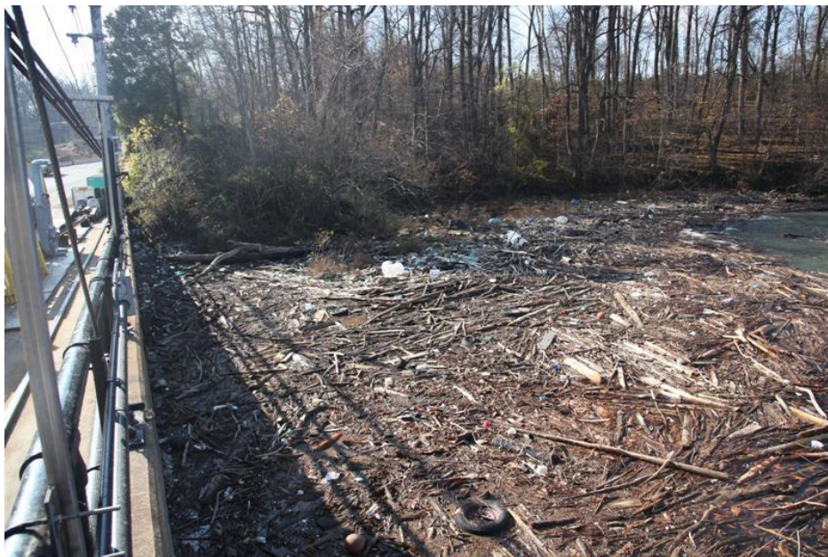
FIGURE 4.1.1-2: ACCUMULATION OF DEBRIS AT THE CONOWINGO DAM INTAKE STRUCTURE
