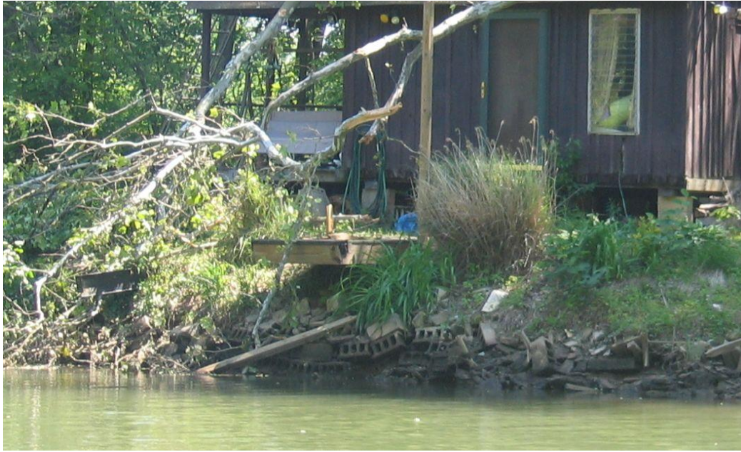
FIGURE 4.1.2-3: COLLAPSING CINDER BLOCK BULKHEAD (MAY 2008)
