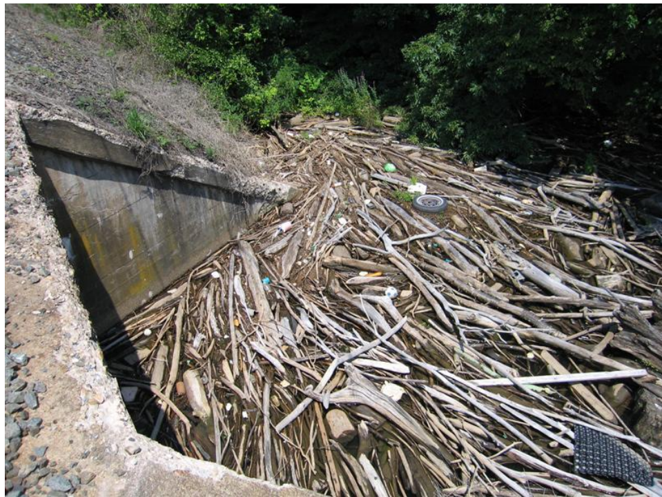
FIGURE 4.1.1-8: CLOSE-UP OF THE TRASH DEBRIS TRAPPED AT CULVERT (JULY 2008)
