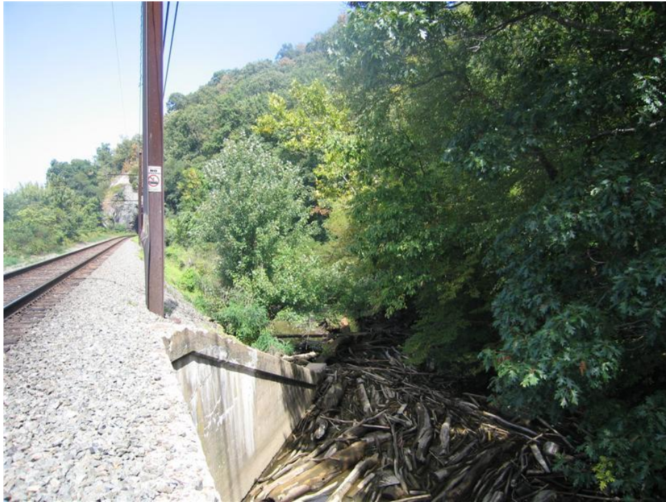
FIGURE 4.1.1-7: DEBRIS BUILD-UP AT TRIBUTARY CULVERT (SEPTEMBER 2007)
