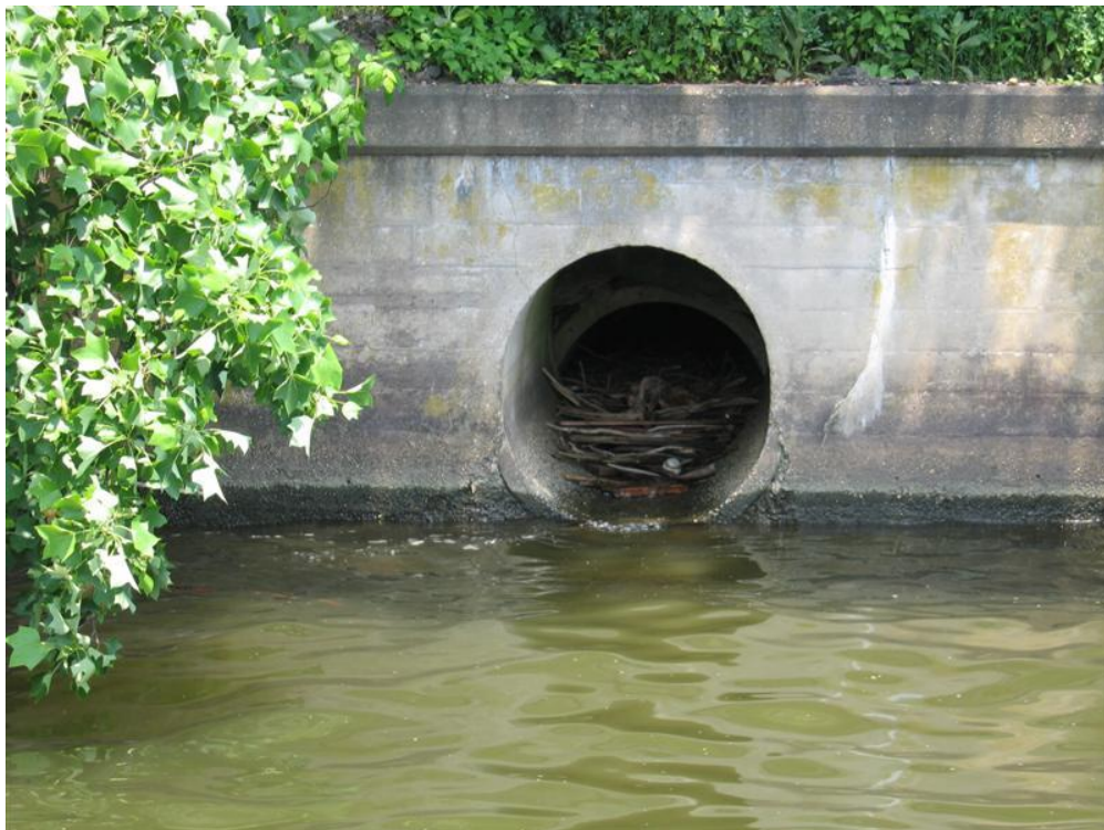
FIGURE 4.1.1-6: DEBRIS BUILD-UP IN SMALL CULVERT (SOFT BALL IN FOREGROUND) (JUNE 2008)
