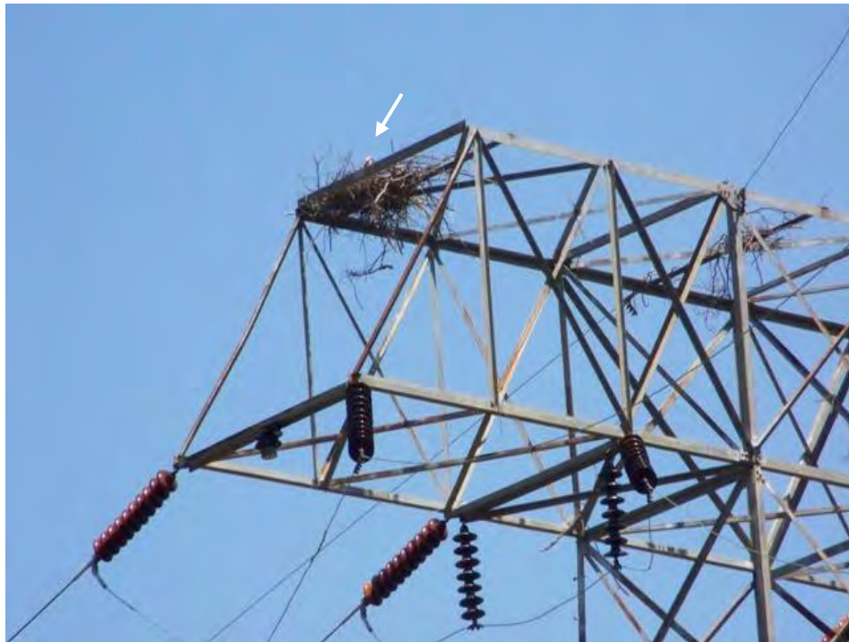
Photo 12: An osprey in incubating position in Nest No. PA-2 high in the crosspiece of a transmission tower on the east side of McCalls Ferry Road in 2010
